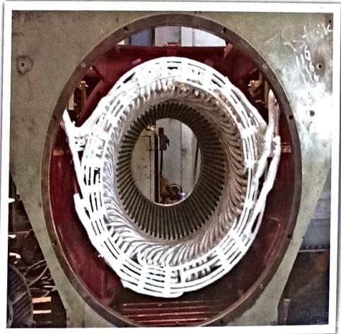
1800 KW, 690 V, VFD Motor stator after rewinding
